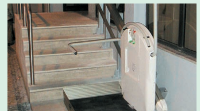
Prestigious office building installation; SW10
